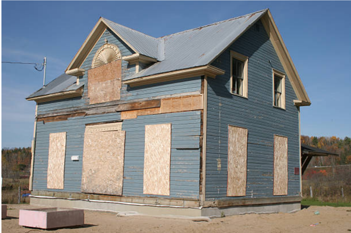
Figure 2.1.1 Houses could have boarded up windows
