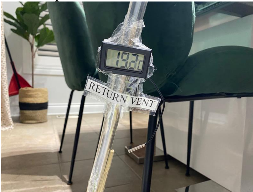
Figure 7. Return vent testing result
