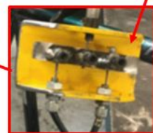
Cable Splitter Box
